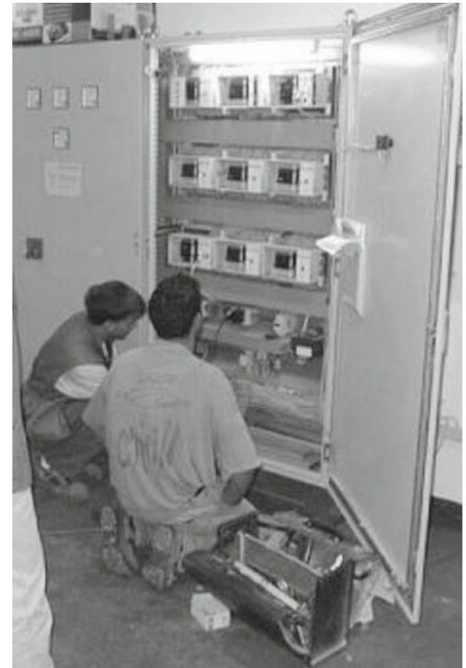
Fig. 1.9 The terminal block and DDCs mounted in a control cabinet [ABB]
