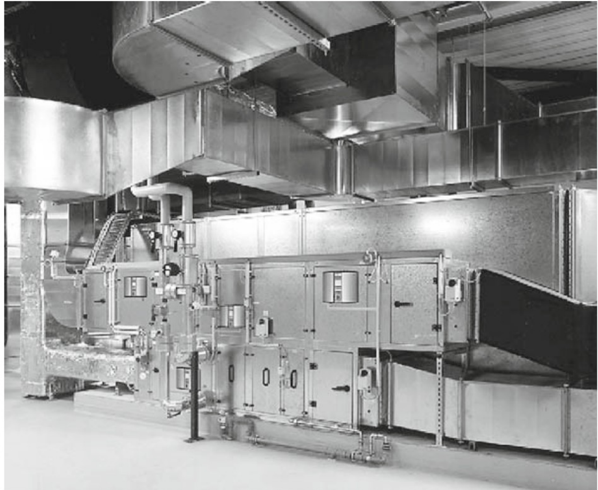
Fig. 1.1 A ventilation system in a commercial building [ABB]
